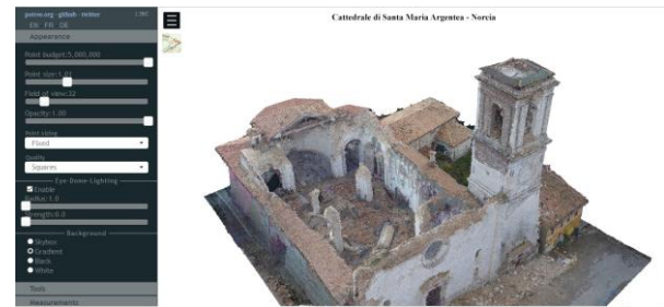
Figure 8. Point cloud of the Co-cathedral of Santa Maria Argentea deriving from photogrammetric UAS survey.
