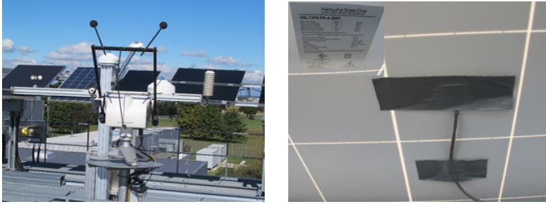
Figure 4: Weather station (on the left) and module temperature sensor (on the right).
