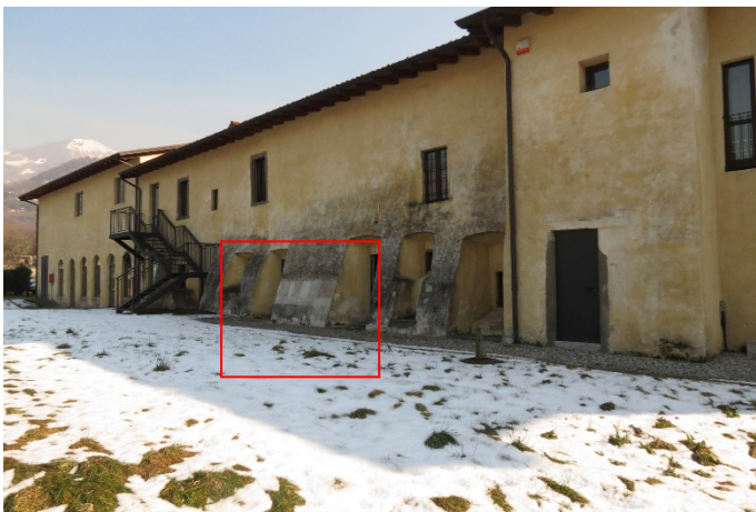
Figure 1 Lavello Convent, Calolziocorte: Northern side. The square frames the areas of application of the biocides under test
