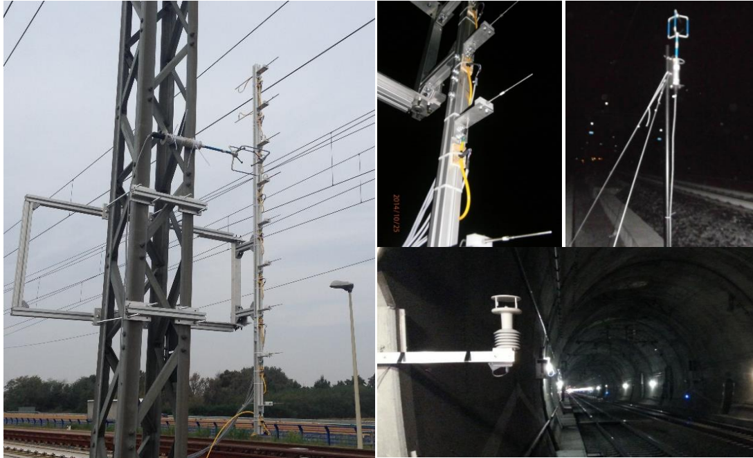
Figure 3: Instrumentation installed trackside: pitot rake, pressure taps and sonic anemometer.
