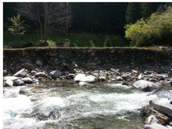
Figure 4. Eroded bank in Tartano basin
