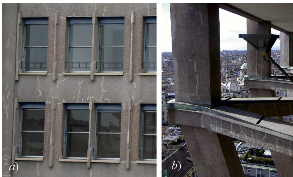
Fig. 2. Details of elements on the facades of Torre Velasca: pillars and beams (a), struts (b).
