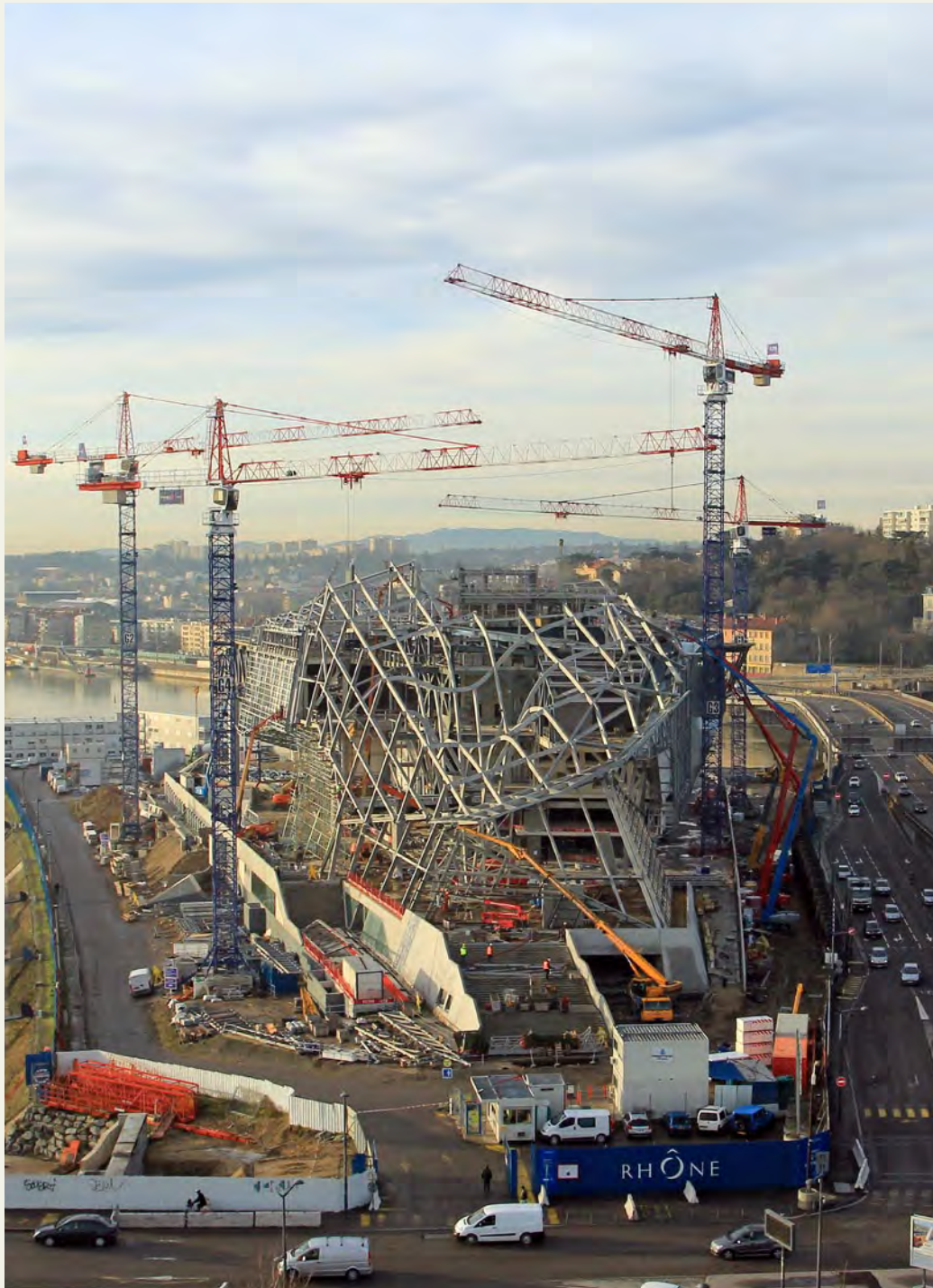
IMG. 2.27 — Musée des Confluences, Lyon, France. Project by Coop Himmelb(l)au. View of the construction site. © Hubert Canet, Balloide Photo.
