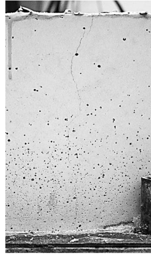
Figure 30b: D5-0.5 ring test crack
