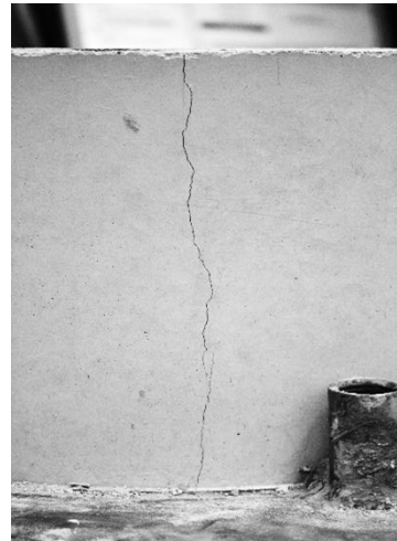
Figure 29b: CM ring test crack
