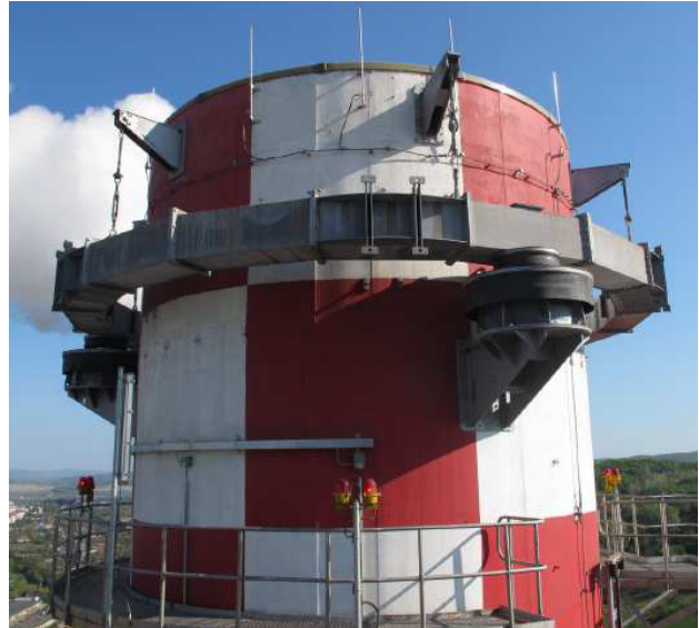
Figure 2. The tuned mass damper after its installation.
