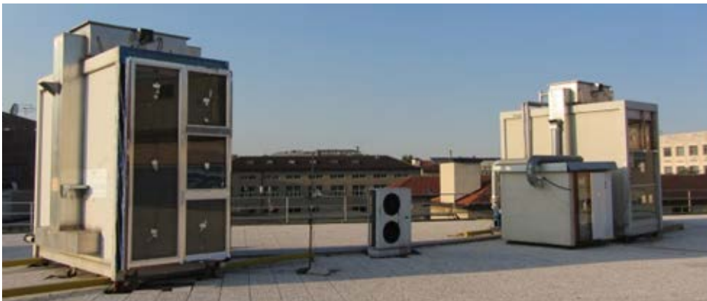
Figure 3. View of the TWINS test facility at Politecnico di Torino
