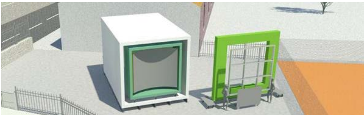
Figure 2. 3D perspective of the new test cell facility under construction at ESTP (Paris)
