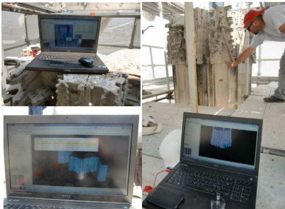
Figure 6. The use of the WEB Bim system in the yard as support for the disassembly of the oldest spire of the Milan Cathedral.
