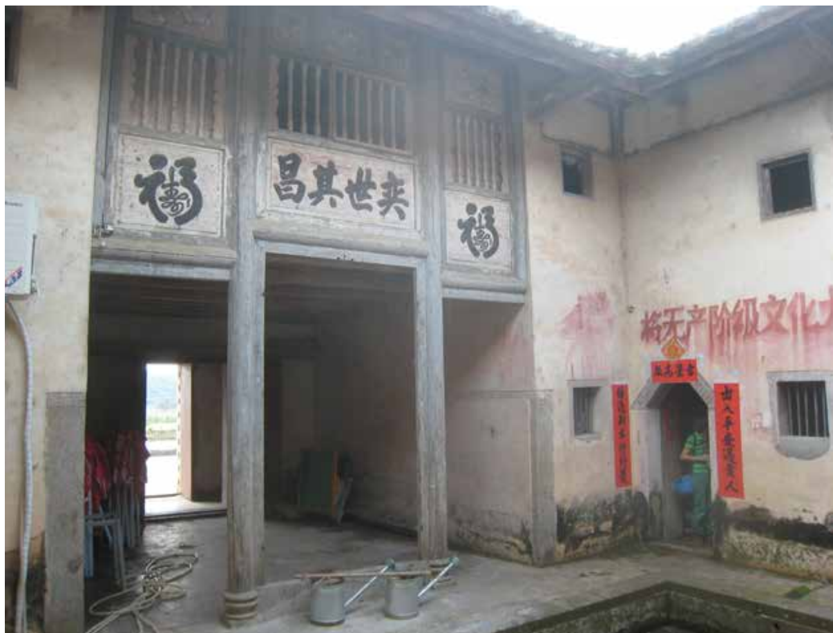
On this page and at pages 46-47: Architectural survey of Hui Xin Lou, residence. (Domenico Chizzoniti, Giovanni Comi, Rossana Gabaglio, Mariacristina Giambruno, Stefano Perego, Zhu Tan with Cecilia Bischeri, Jiang Weiwei, Liu Xiaoxiao, Giacomo Menini, Fabio Zangheri, Lucilla Zanolari Bottelli, 2010).
