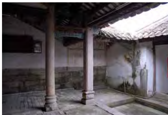
In this page and at page 53: Architectural survey of Jiang Tian Nan Yang Shi Ju residence. (Domenico Chizzoniti, Giovanni Comi, Rossana Gabaglio, Mariacristina Giambruno, Stefano Perego, Zhu Tan with Cecilia Bischeri, Jiang Weiwei, Liu Xiaoxiao, Giacomo Menini, Fabio Zangheri, Lucilla Zanolari Bottelli, 2010).
