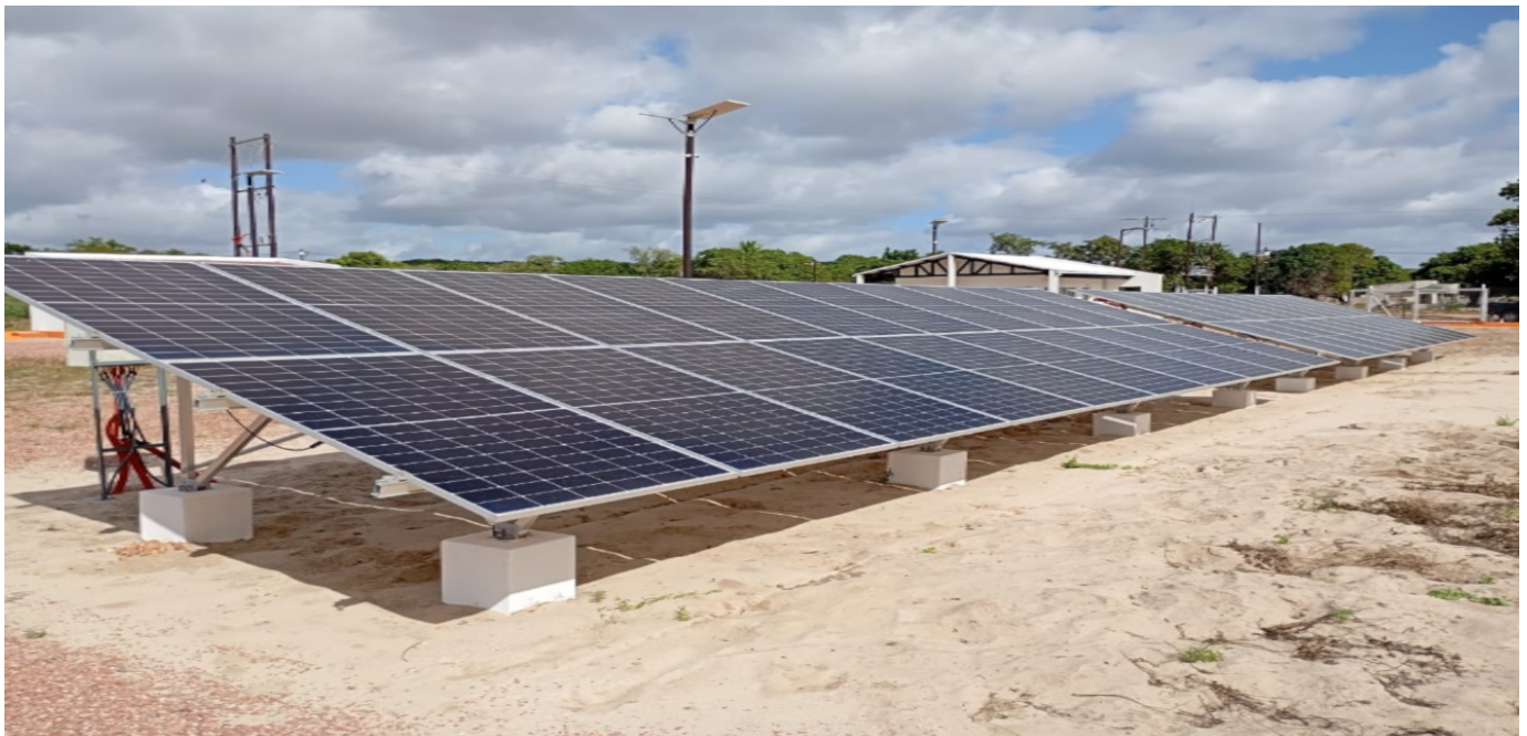
Figure 5. Solar PV system in Mawayela village (photo by the authors).
