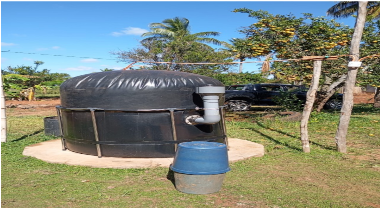
Figure 7. Photo of HB system in Dongane village (photo by the authors).
