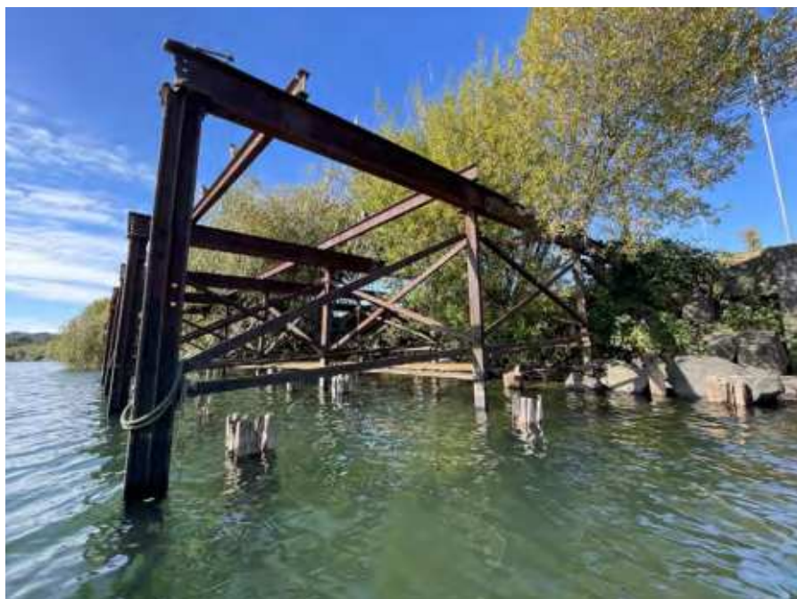
Fig. 5 – Vestiges of a river jetty (photo by ECJ, 2023).
