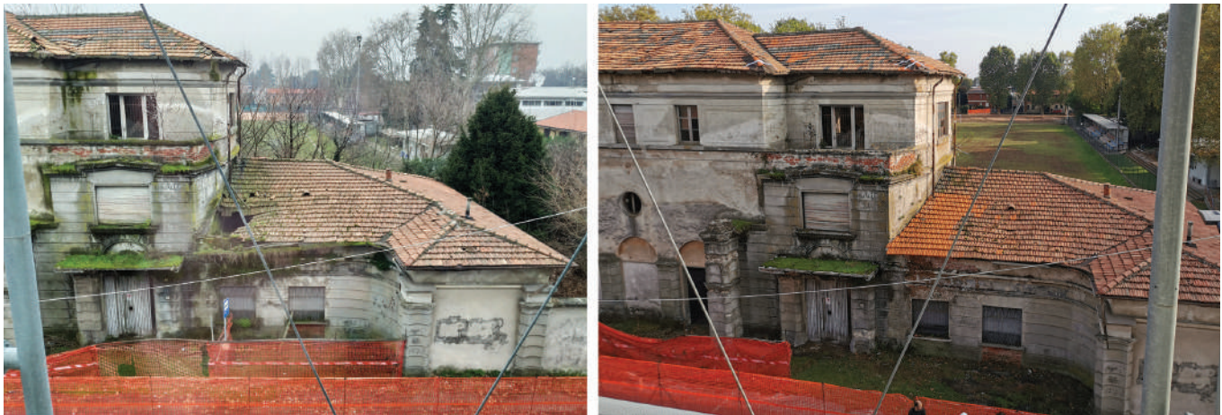
Figure 6. Roof photo of the north side towards the west corner before (left) and after (right) the urgent repair works in 2020. The 3-types of tiles are easily recognizable: the oldest dark ones, the new brilliant red ones and the other dull red ones.
