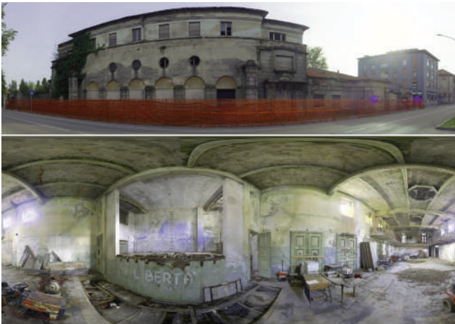
Figure 4. TLS panoramic images of the north facades and of theatre in the inner salon.
