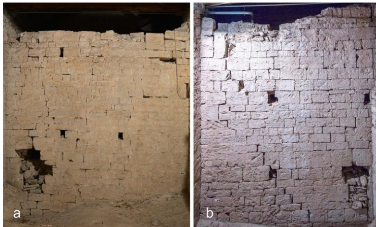
Fig. 2a 2b – The cracks observed on the surviving parts of the ancient bell towers(author).
