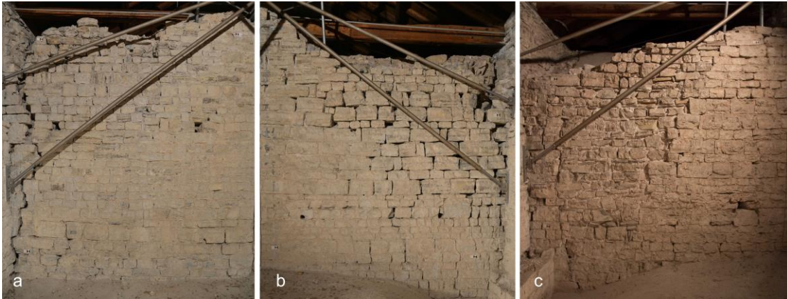
Fig. 1a, 1b, 1c, - Damage on the north and south facades of the transept. Please note in picture 1c the rebuilt part with a later crack on the left side (author).
