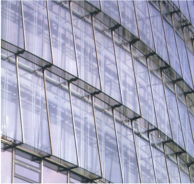
Fig. 11 Helmut Jahn, Post Tower , Bonn. Segmented external shading skin (south elevation), framed by linear vertical and horizontal aluminium profiles, that creates a visual and functional membrane to the internal curtain wall © Courtesy of Helmut Jahn
