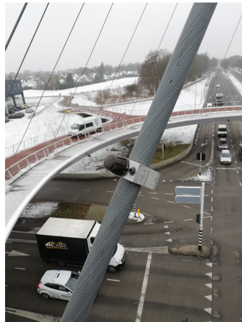
Figure 5: The Lord G-Link 200 accelerometer installed on the cable.
