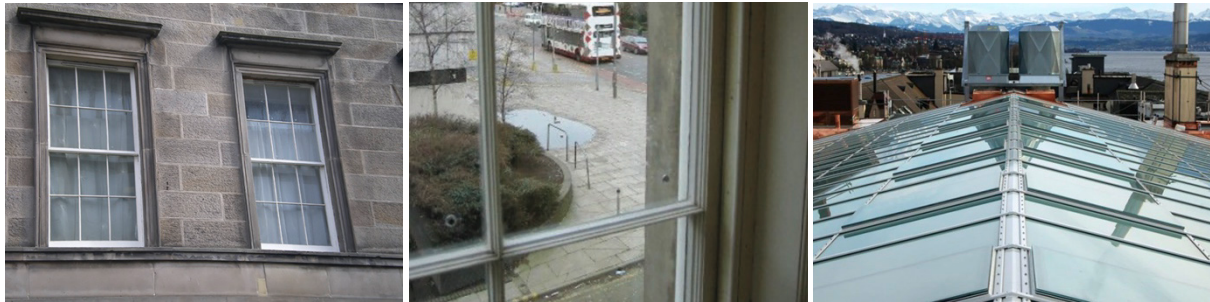
Figure 3 (a, b). Vacuum glazing installed in a historic building located in Edinburgh. Source: [17]
