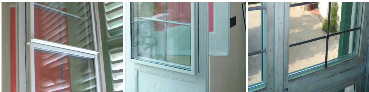
Figure 2. Example of installation of a secondary external glazing in Villa Piazzi in Nerviano (MI) by the restorer Ercole Livio Rini. (a, b) View of the external side. (c) Inside view of the closed window.
