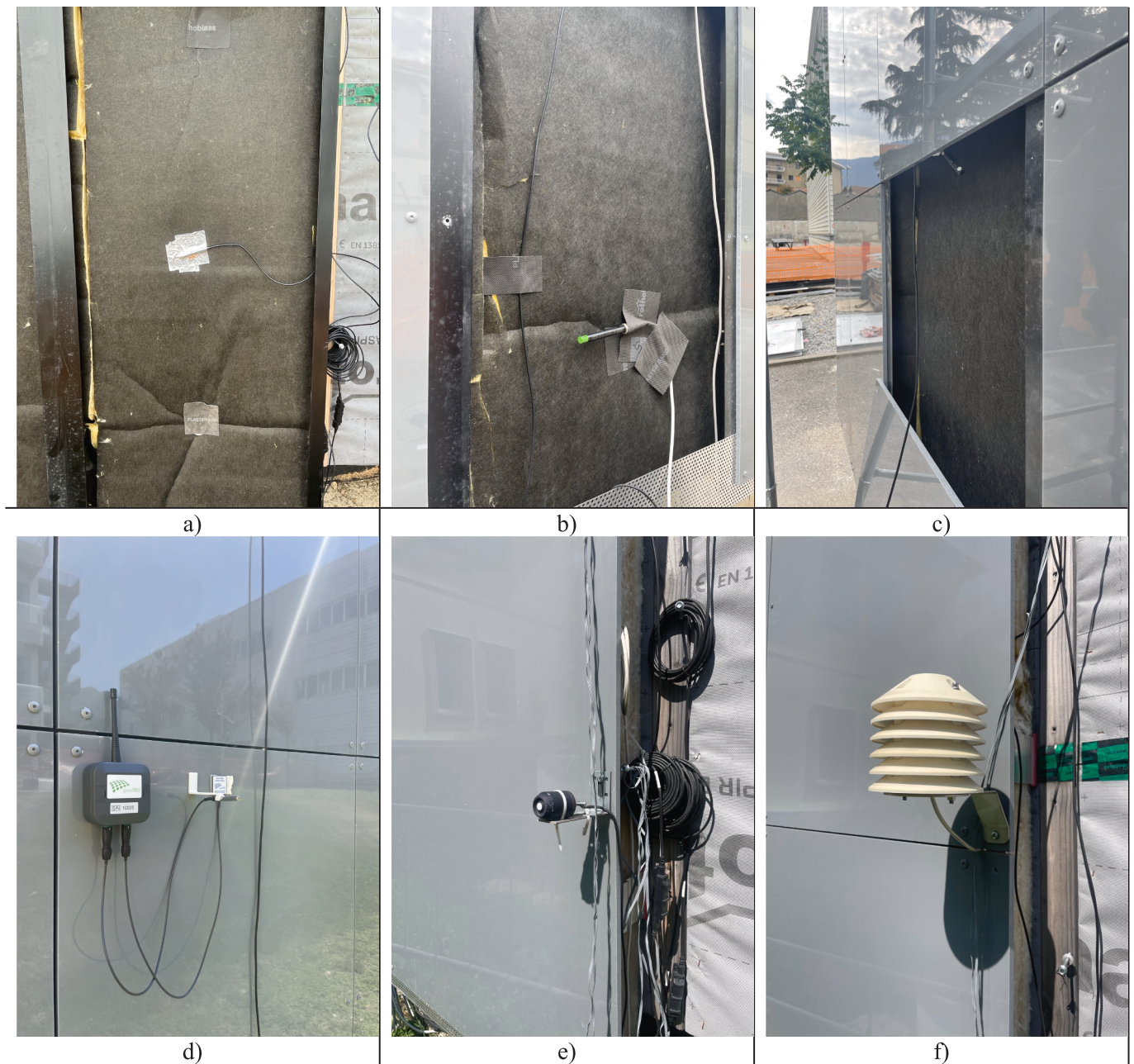
Fig. 11. Pictures of the sensors mounted on the OVF: a) surface temperature sensor on the external surface of the thermal insulation layer; b) air velocity sensor inside the OVF cavity; c) air temperature and air humidity sensor inside the OVF cavity; d) surface temperature sensor for the cladding temperature monitoring; e) global solar radiation sensor on the facade; f) air temperature and humidity sensor located 15 cm from the OVF and 1.5 m from the ground level.
