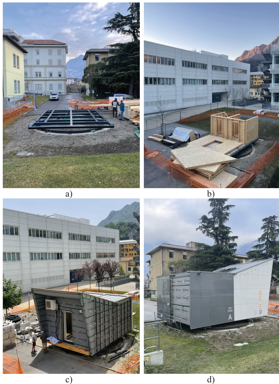
Fig. 5. Pictures of BEE Lab construction phases: rotating steel platform installation (a), prefabricated wood-based envelope assembly (b), ventilated facade installation (c), completed lab (d).
