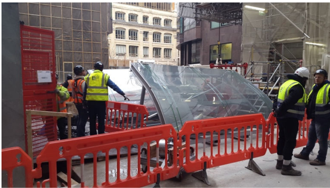
Fig. 16. Fletcher Priest Architects, Angel Court Building , London (© Courtesy of Focchi).
