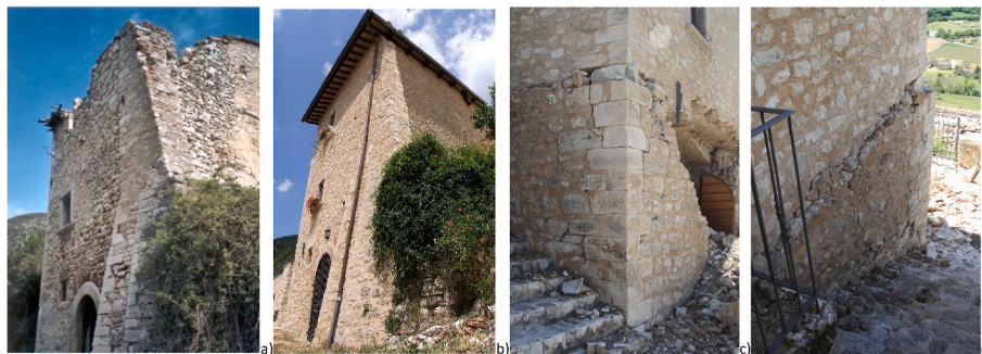
Fig. 5. Photos of the case study in Campi Alto di Norcia: a) after the 1997 earthquake; b) after 2000s restoration; c) and d) after the 2016 earthquake: overturning out-of-plane of the ground floor facade and rigid rotation of the renovated upper volume.
