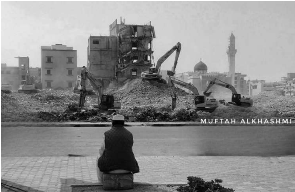
Figure 5. The start of the demolition of Benghazi's historic center. (Photo by Muftah Al Khashmi, 2023)
