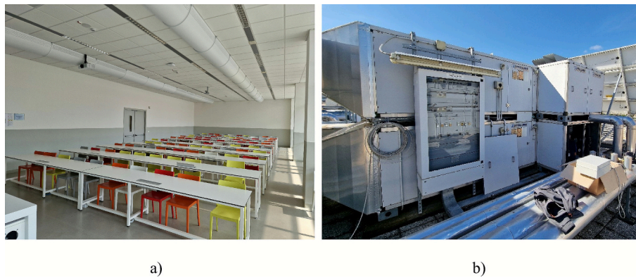
Fig. 3. A) view of the monitored classroom; b) view of the ahu serving the classroom located in the rooftop.
