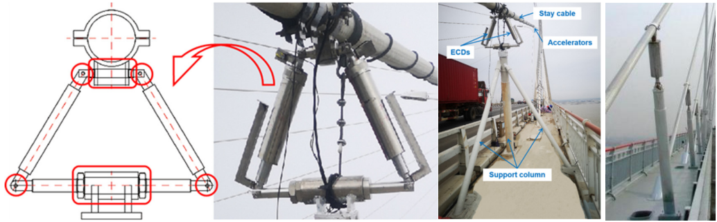
(a) Eddy current damper system (ECDS), (b) Original stay cable damper system
