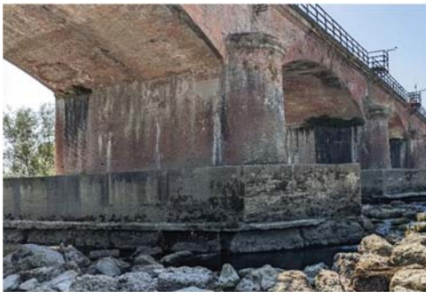
Fig. 5. Foundation scour at pier P08 (picture from the upstream side).
