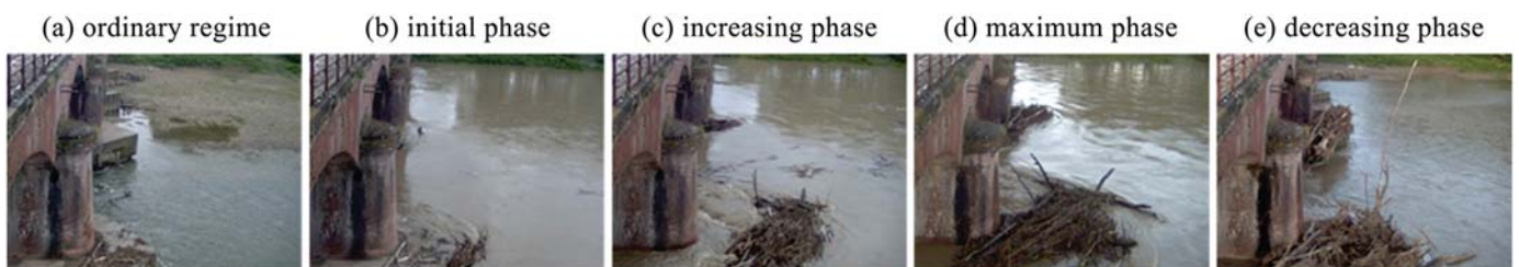
Fig. 15. Debris accumulation process at pier P05 on May 12th, 2021.
