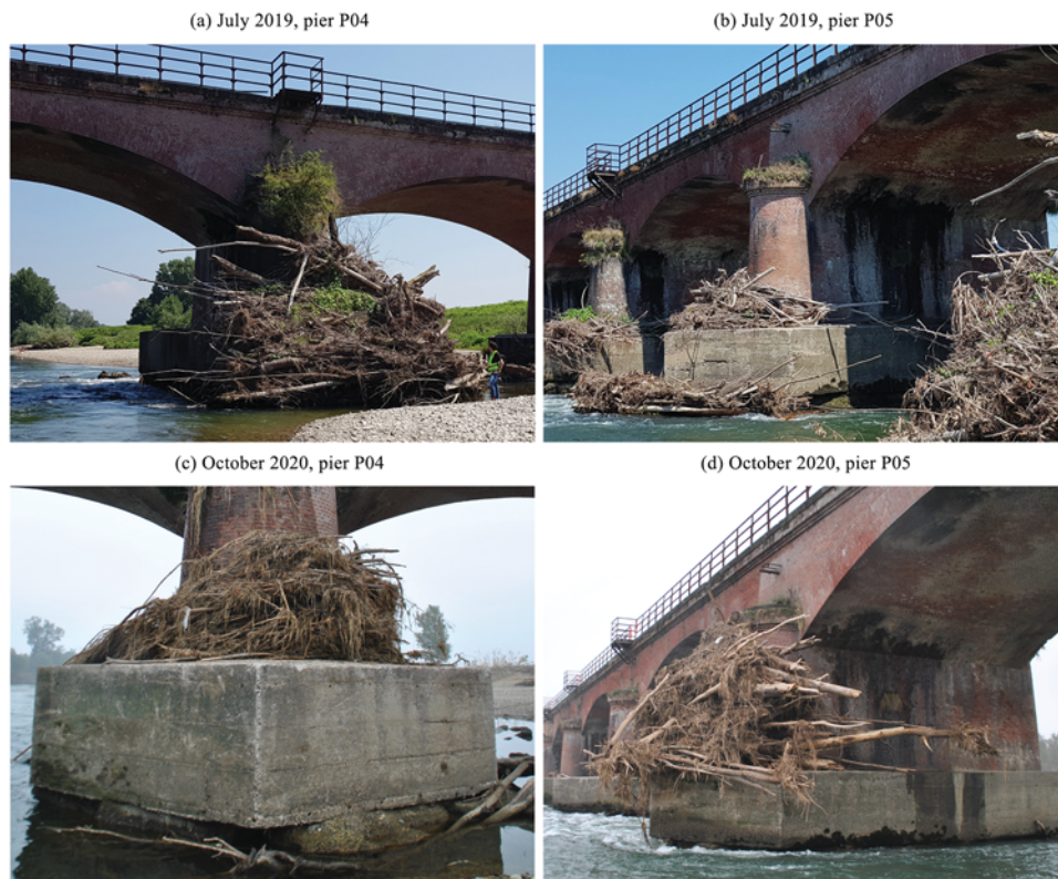
Fig. 2. Variations of debris accumulation on piers P04 and P05 before and after the flood of October 2020.
