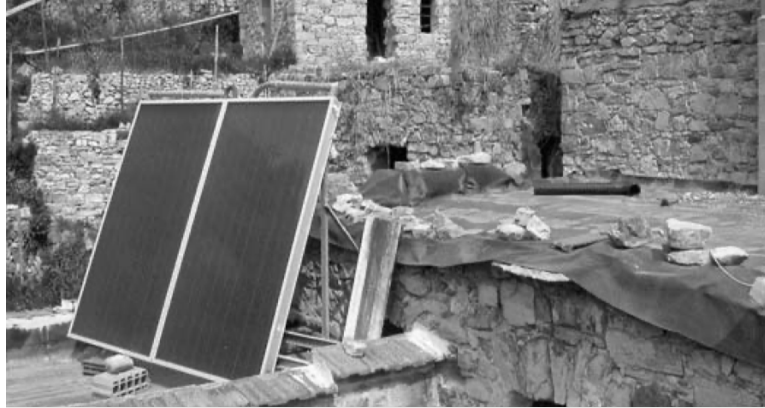
Fig. 3.63 Solar panel in the Torri Superiore eco-village 85
