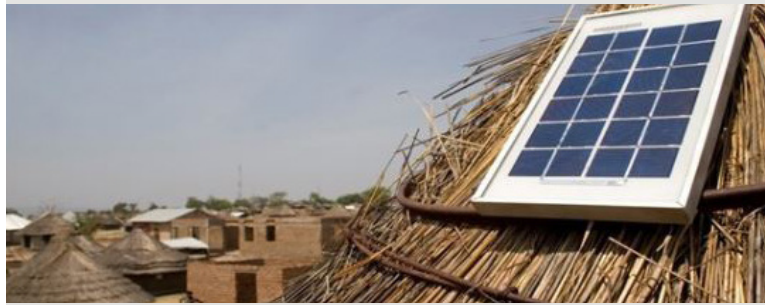
Fig. 3.74 Solar panel installed on the roof of a rural settlement 96
