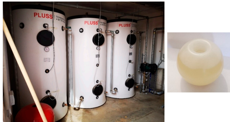
Figure 5. Heat storage tanks ( 3 \times 1000 L) and a PCM module.
