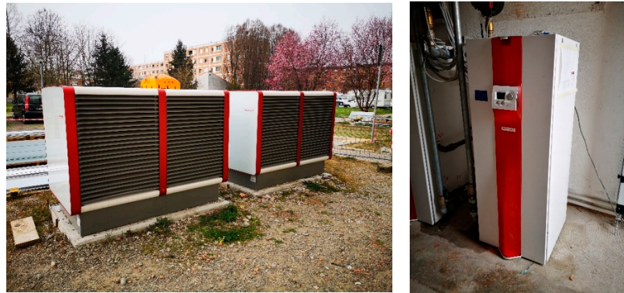
Figure 3. Outdoor and one of the indoor heat pump units.
