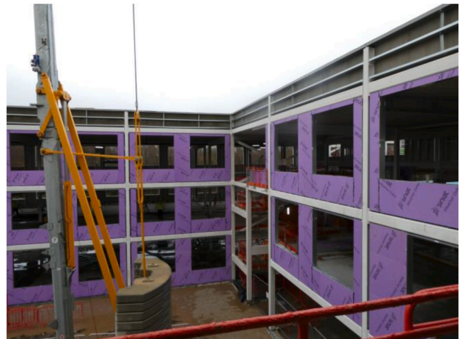
Fig. 4. Pre-assembled lightweight exterior infill wall panels installed in the primary structural frames.
