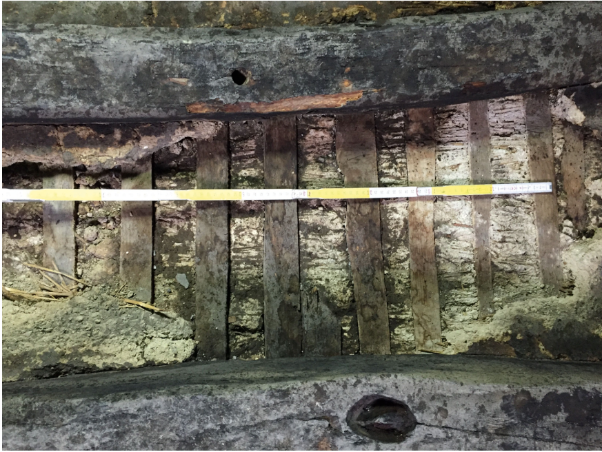
FIGURE 8 Partially removed upper part of mortar plus straw. The laths net between the beams and the top part of the plastered ceiling are visible.
