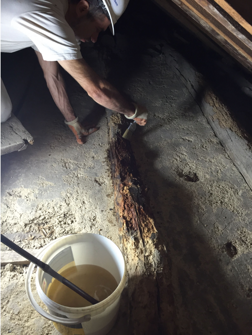
FIGURE 19 Punctual consolidation is done by brushing the deteriorated sapwood with liquid resin.
