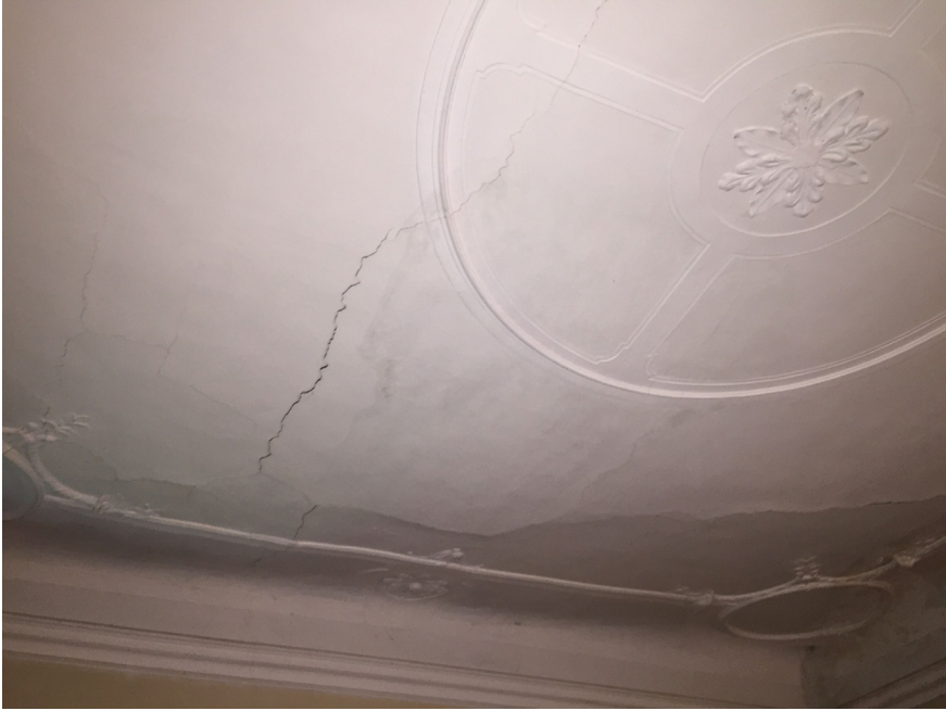
FIGURE 10 View of the ceiling of a room with bending, cracks, and detachment of the ceiling plaster
