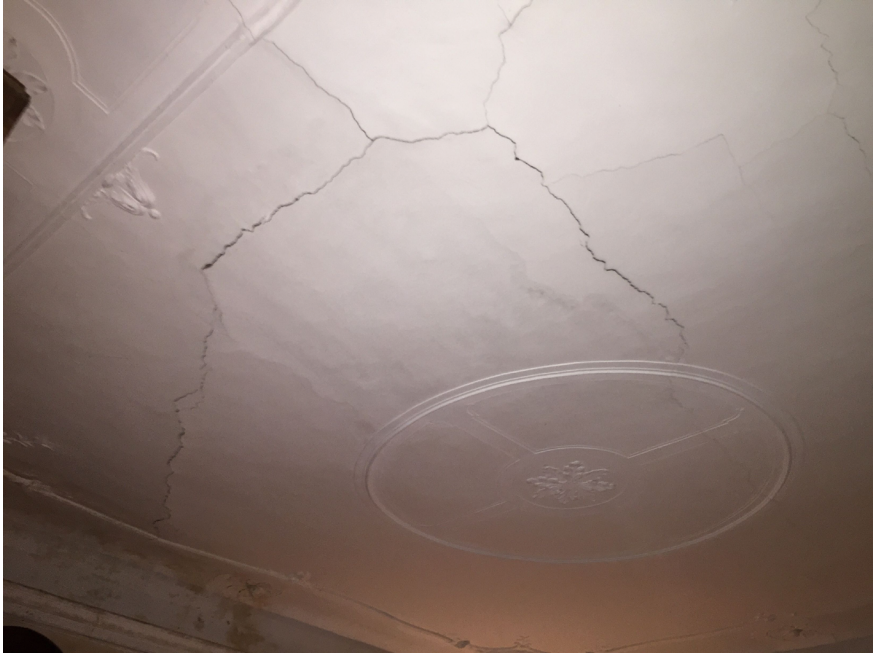
FIGURE 11 View of the ceiling of a room with bending, cracks, and detachment of the ceiling plaster
