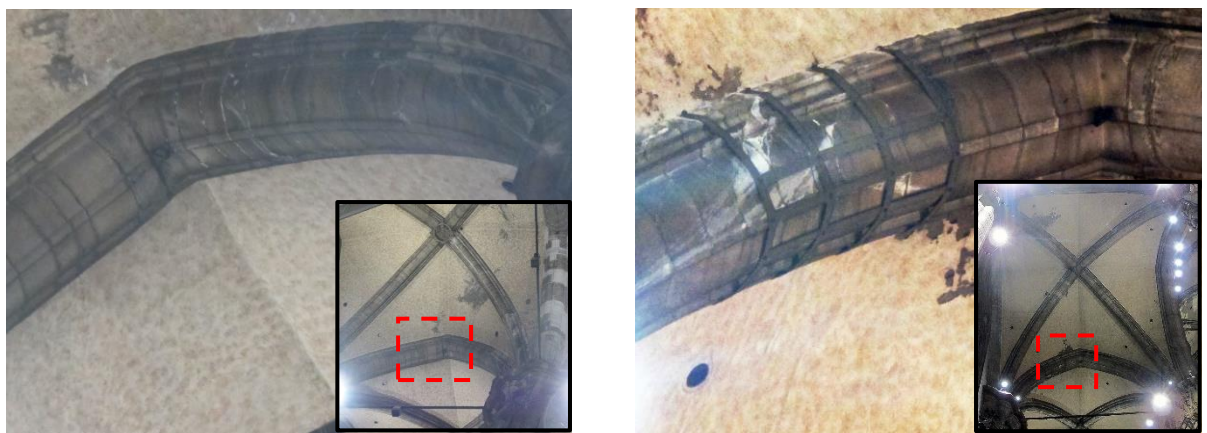
Figure 4. a) Distorted arch observed in the vault 113, b) Strengthening observed today in the vault 119, symmetrical to vault 113 with respect to the cathedral longitudinal axis.
