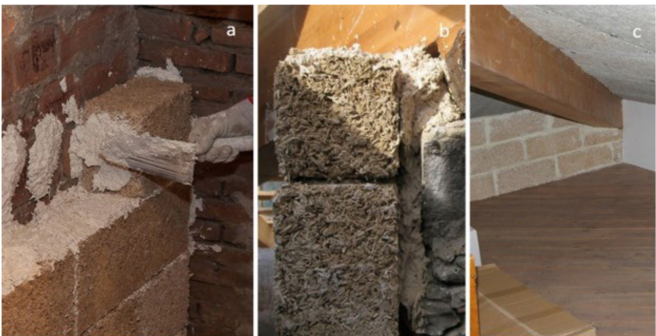
Fig. 3.9-5 Details of non-load-bearing walls made of hempcrete blocks: (a) wall erection; (b) side view; (c) front view
