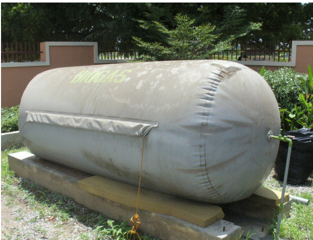
Fig. 6.4-16 – Above ground plastic inflatable gasholder
