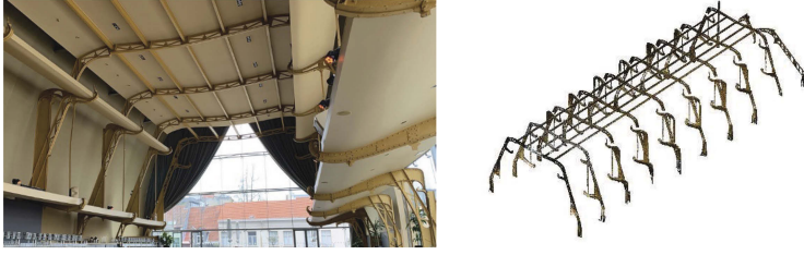
Figure 2. Café Horta, interior view (left), captured point cloud after steel segmentation (right).
