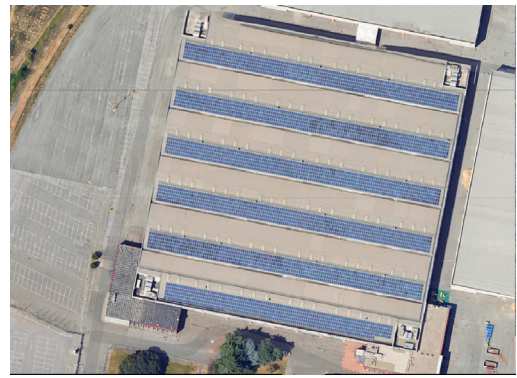
Fig. 1. The PV system under investigation from which the EL images from the PV modules were captured.
