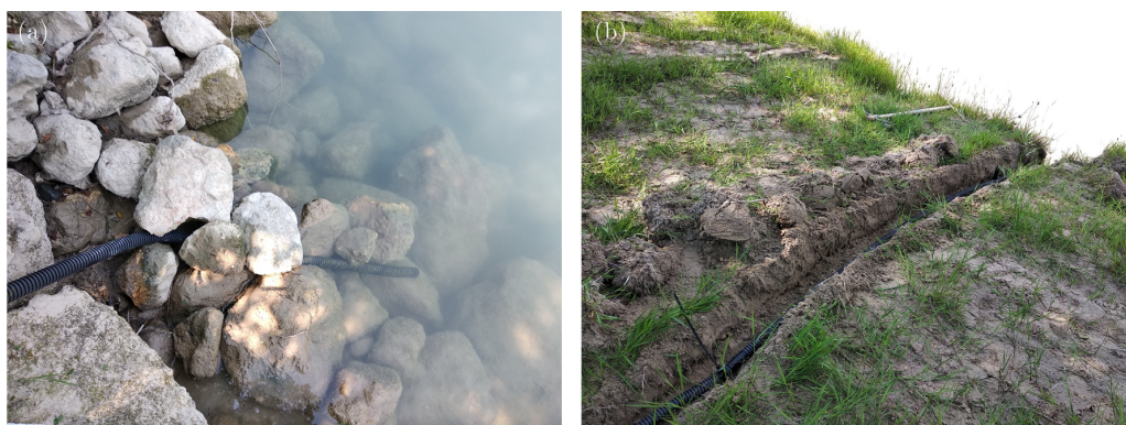
Figure 4. Water level sensor installation in the main channel: (a) Upstream section—the tube is surrounded by rocks. (b) Downstream section—the tube is buried within the river bank.
