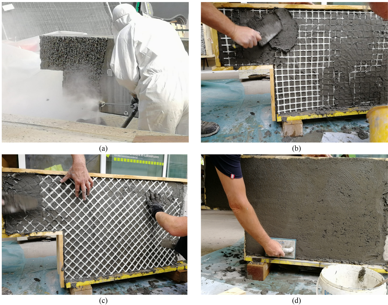
FIGURE 10 Application of the FRCM retrofitting system on the RC dapped-end beam: hydro-scarification of RC beam surface (a), placing of the fabric layer at 0^\circ (b), placing of the fabric layer at 45^\circ (c), and cast of the finishing layer (d). FRCM, Fabric-Reinforced Cementitious Matrix; RC, reinforced concrete.
