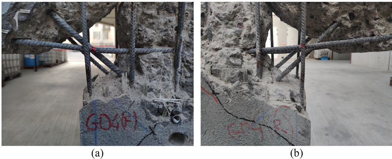
FIGURE 21 Detail of the rebar rupture in specimen RTF-(0°)-01 after concrete demolition: failure of the U-shaped horizontal bar on the front side (a), and of the first stirrup on the back one (b). Note that the latter view is reversed.
