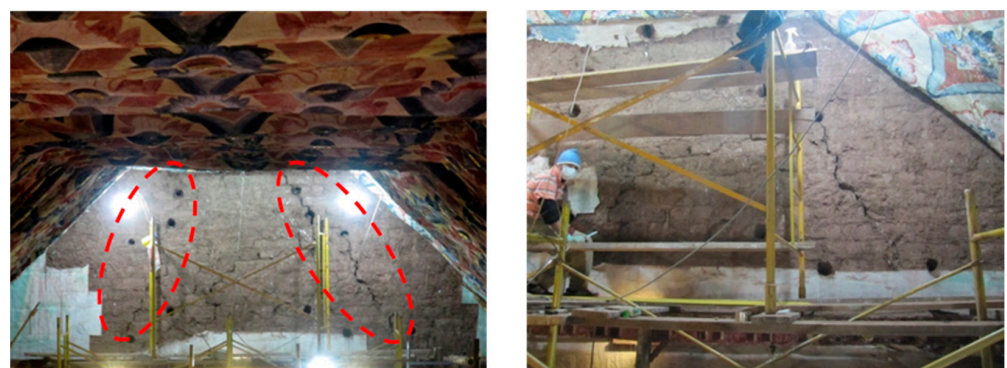
Figure 16. Damage to the triumphal arch of the Church of Andahuaylillas (reproduced from [50]).
