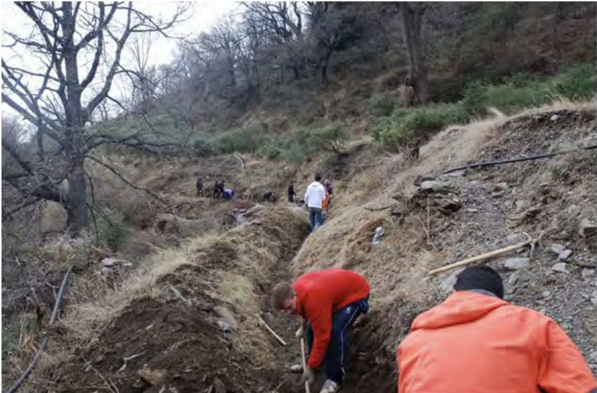
Fig. 11. Restoration of the Barjas irrigation channel in Cádiz, Southern face of Sierra Nevada (Granada)
