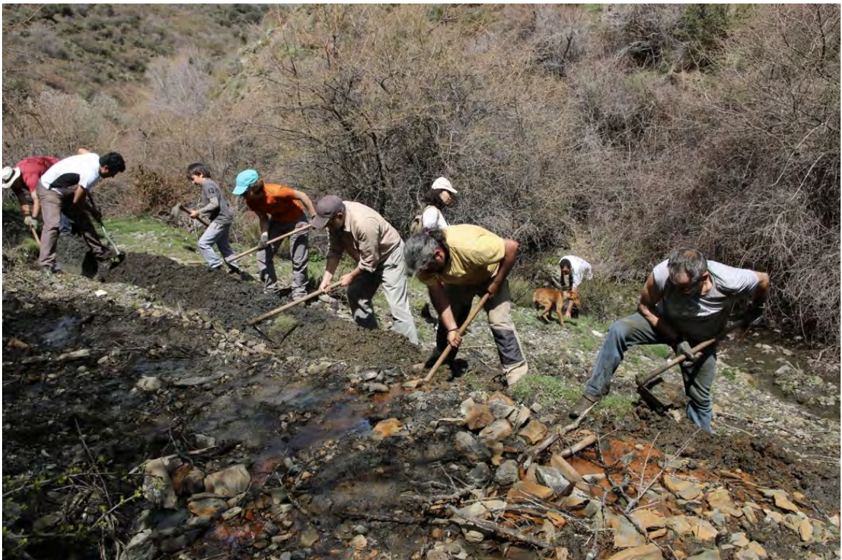
Fig. 10. Restoration of one of the careo channels in Lugros, Northern face of Sierra Nevada-Granada
