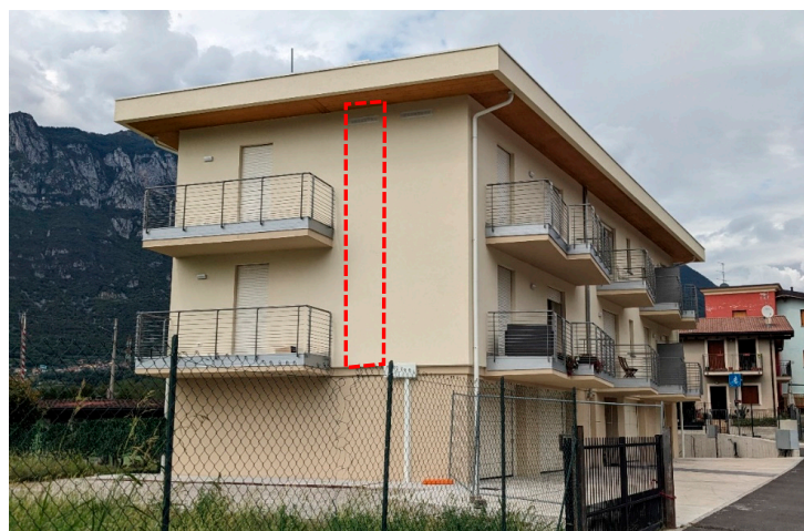
Figure 2. Monitored building, and illustration of the TCC ventilated envelope area analyzed (red dashed box). © Pastori S.
