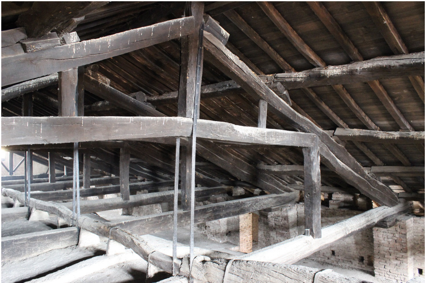
Fig. 7. Unmodified truss of the second phase: T8 truss seen from the north-west. (Photo by Emanuele Zamperini).
