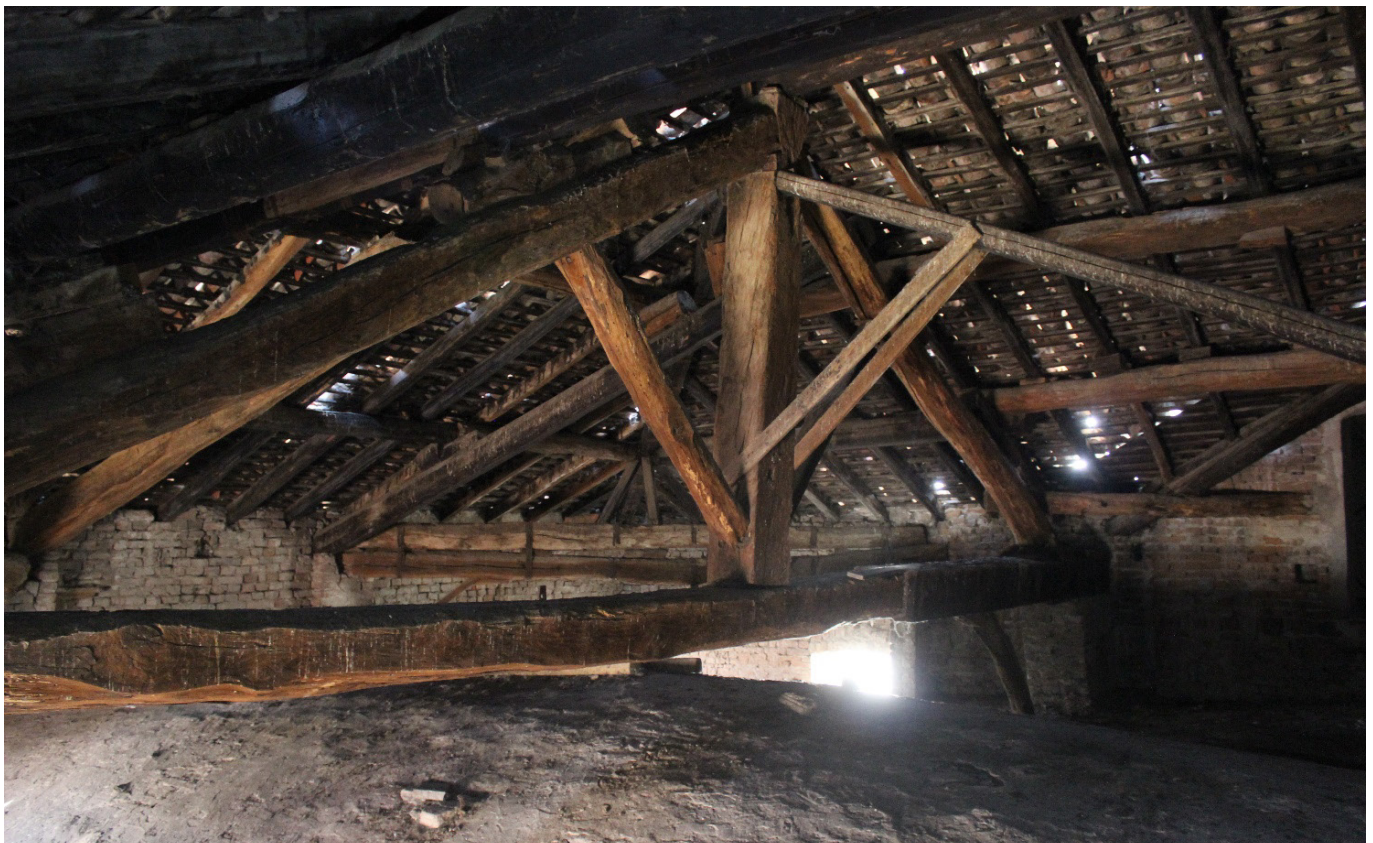
Fig. 3. Closed joint king post truss in the attic above the presbytery of the church. (Photo by Emanuele Zamperini).
