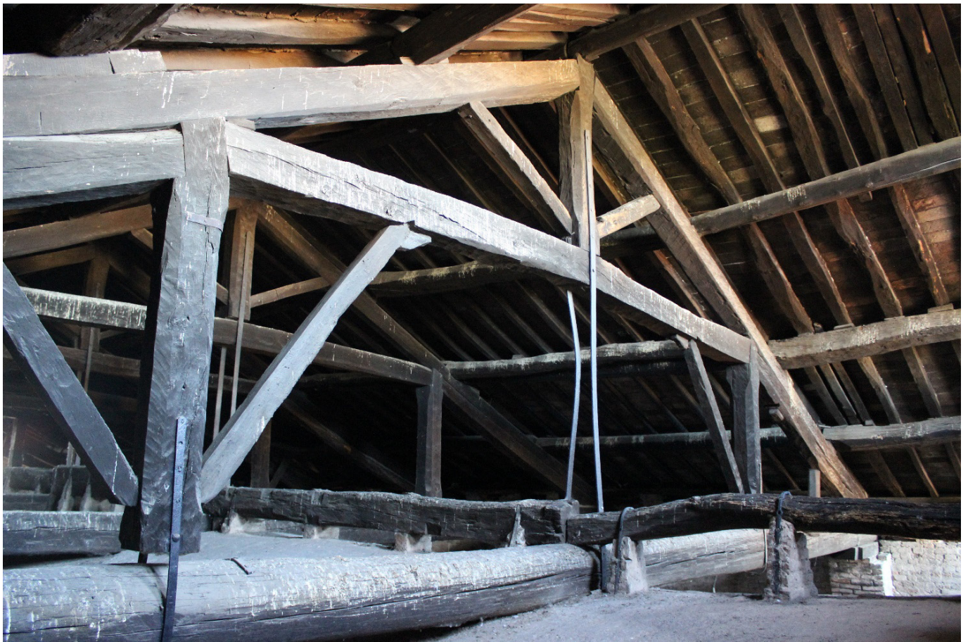
Fig. 9. Modified truss of the first phase: T2 truss seen from the south-east. (Photo by Emanuele Zamperini).
