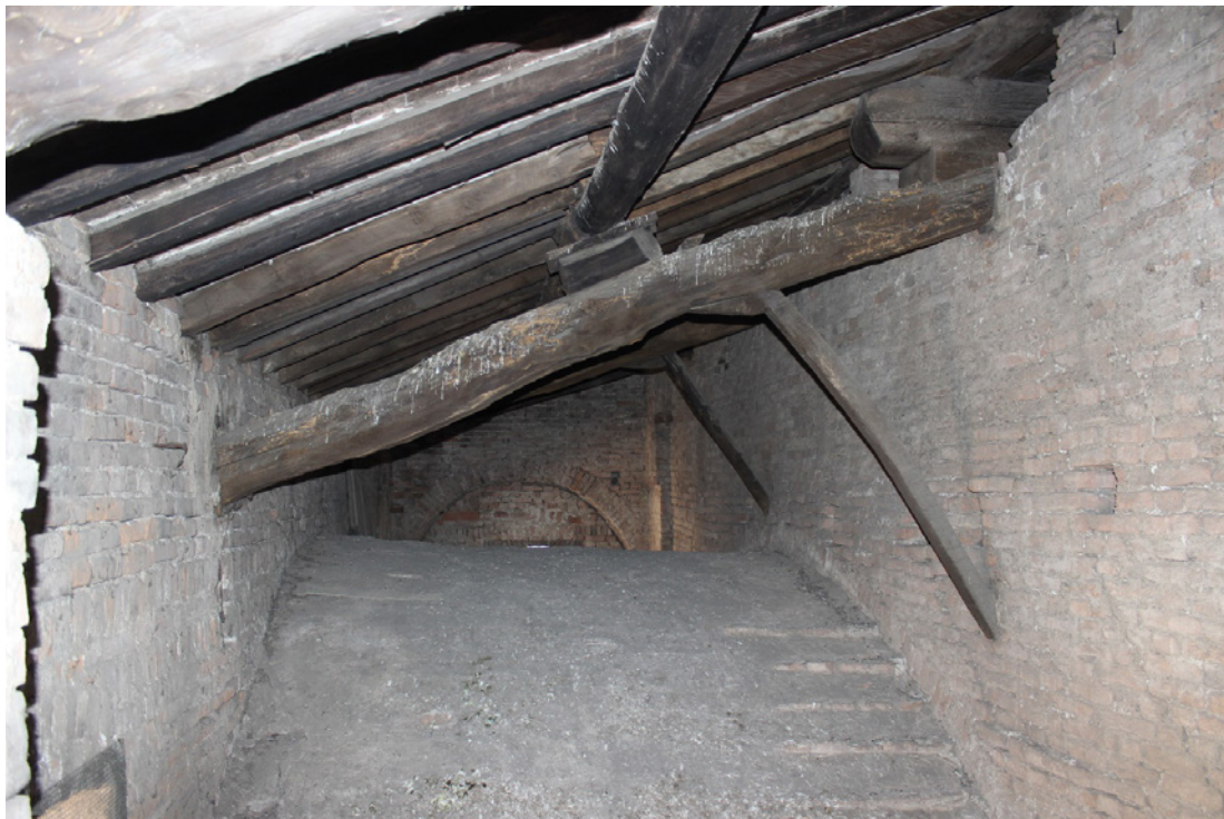
Fig. 4. Roof of the band on the northern side of the nave; it is possible to see the extrados of the barrel vault of the pseudo transept. (Photo by Emanuele Zamperini).
