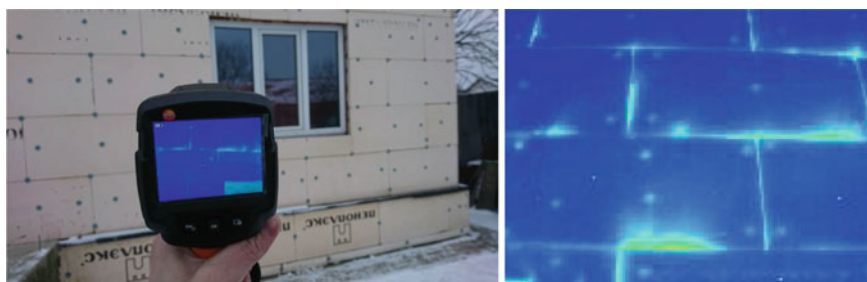
Fig. 1 Thermal imaging of the insulating shell: “bridges” of increased heat transfer are visible
