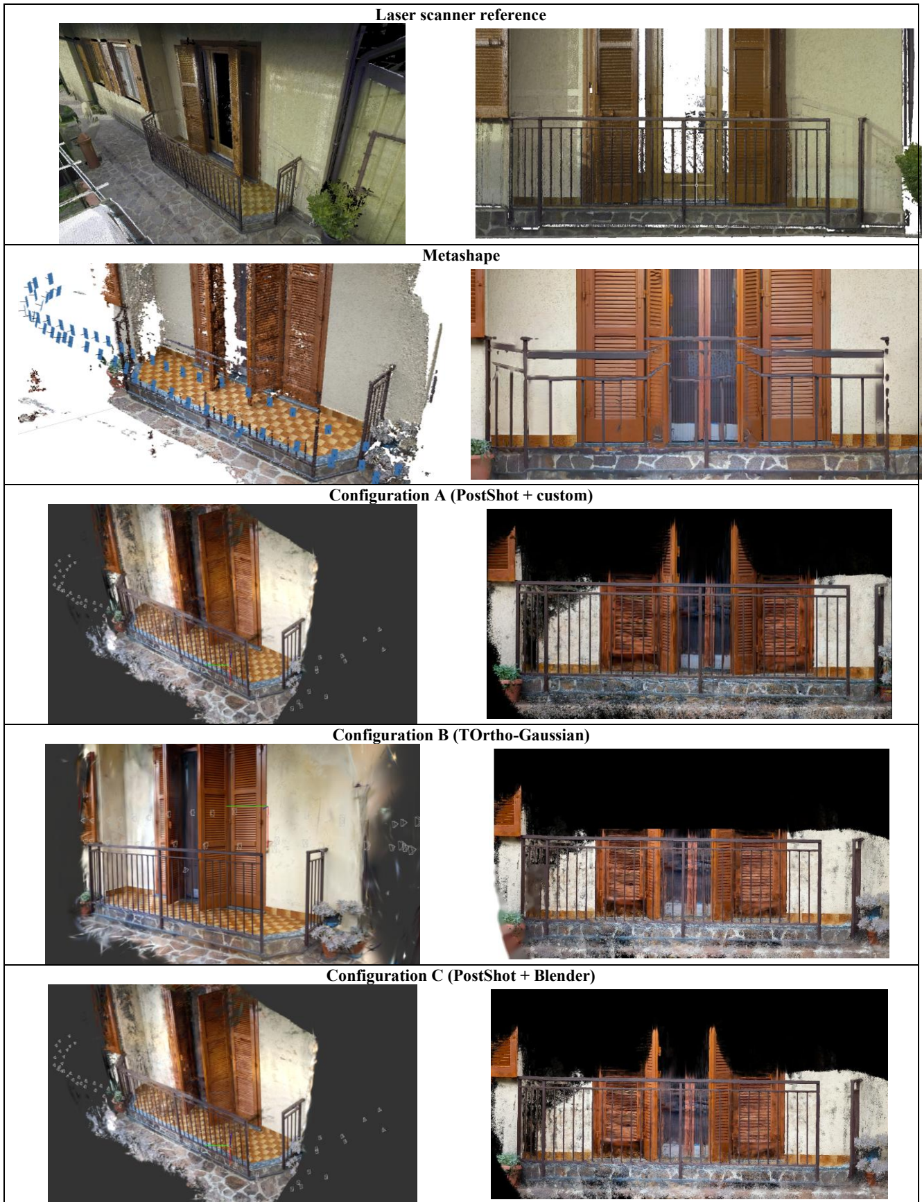
Figure 3. Laser scanner reference and results of the reconstruction of the railings for the different tests: 3D model (left) and detail of the orthophoto (right)
