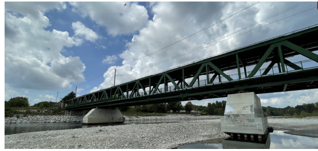
Figure 1. Side view of the actual bridge spanning Ticino River between the municipalities of Turbigo and Galliate.
