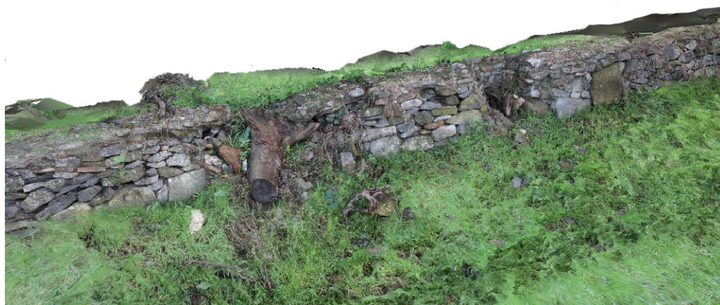
Figure 11. The Macére : a detail of the 3D textured model documenting a portion of the masonry wall damaged with clashed portions and vegetation.
