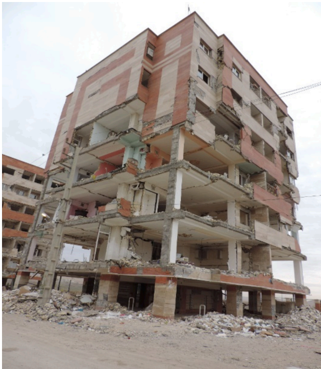
Fig. 1. Extensive damage to the non-structural components of a building after the Kermanshah 2017 earthquake, Iran (picture taken by one of the authors).
