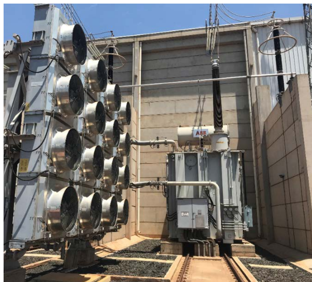
FIGURE 11. Oil to air cooler bank installed in an inverter station.
