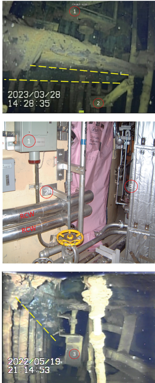
Fig. 18. Erosion height gradients and state of the structures on the outer sides of the pedestal opening (covered by a pink sheet in the central picture); yellow lines mark parts considered to be remaining concrete below the shelves; numbers in red circles indicate original structures that could be identified.
