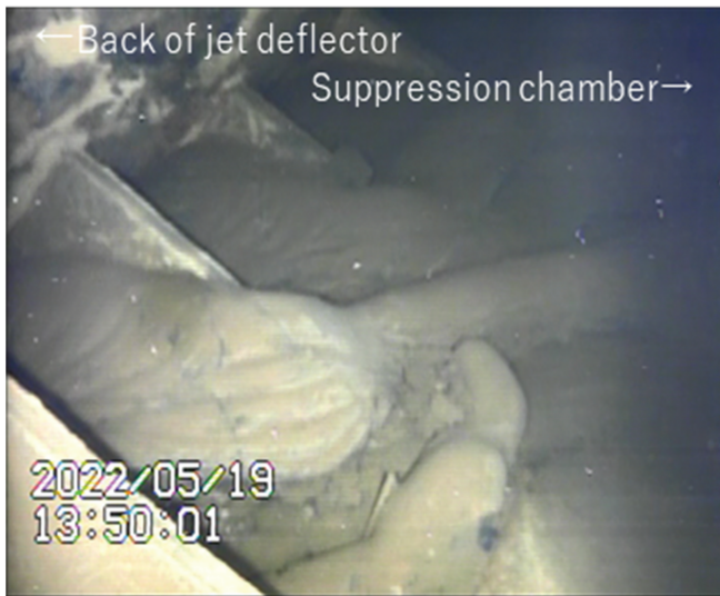
Fig. 14. Clogging of the bottom openings of vent pipe behind jet deflector E (ENE-6).
