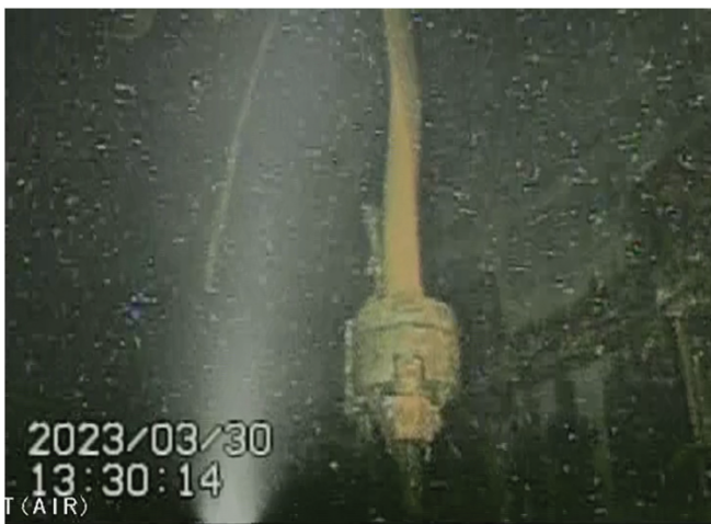
Fig. 5. Detached ICM housing suspended above the water level (SE-3) near the pedestal wall.
