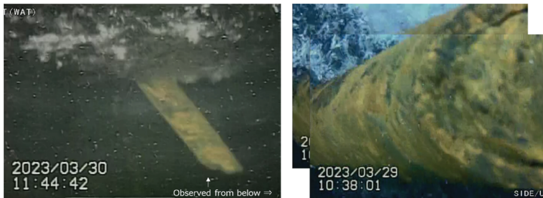
Fig. 8. Clogging of severed CRD housing (central section of the pedestal area) observed from below the severed section of the suspended CRD housing (right picture).
