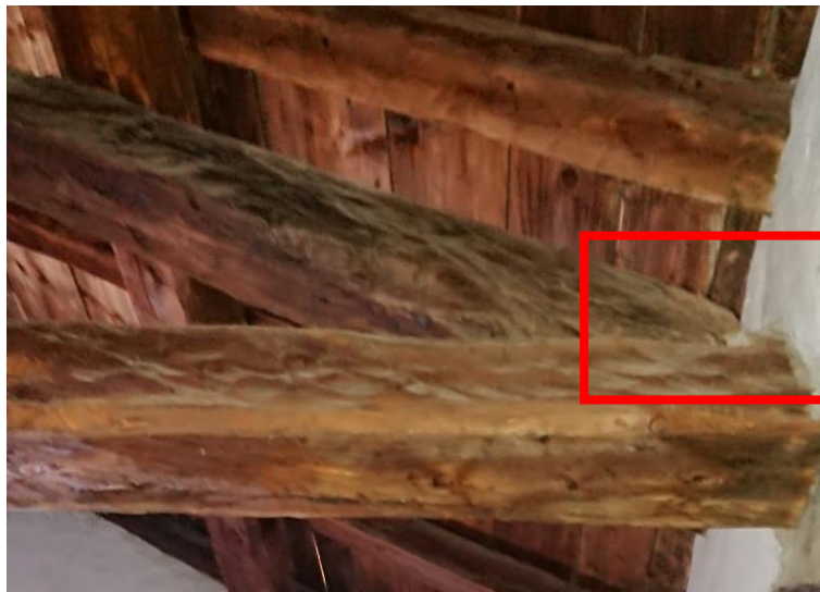
Figure 5: Location of the internal probe, placed on the truss.
