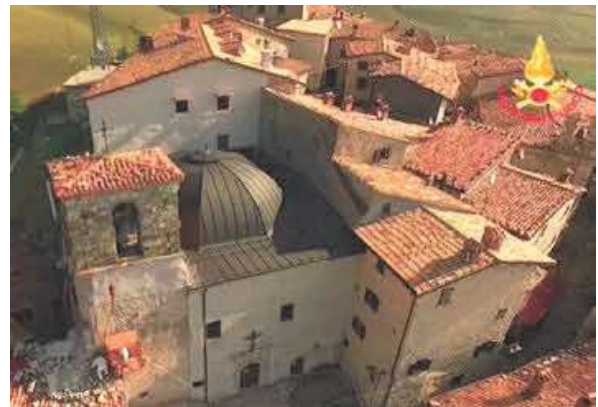
Fig. 5. The provisional intervention on the bell tower of Santa Maria Assunta , realized by the MiC and the NFB (© Vigili del Fuoco ) (Source: https://www.vigilfuoco.tv/umbria/perugia/noceria/messa-sicurezza-chiesa-smaria-assunata ).
