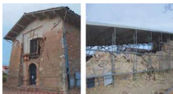
Fig. 3. The church of S. Antonio Abate after the earthquake of 24 th August 2016 (left) and in 2017, after its collapse (right) (Source: https://frascarodinorcia-noprofit.webnode.it/galleria-immagini/ (a); https://www.iluoghidelsilenzio.it/frascaro-norcia-pg/ (b)).
