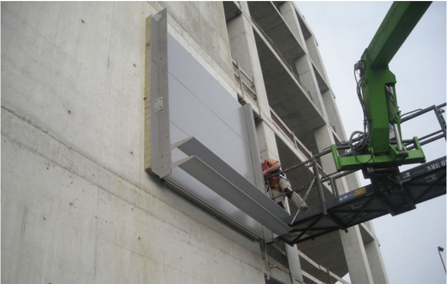
Fig. 1.20 Giancarlo Marzorati, Colour Building , Milan. Construction procedure of the unit components as cladding for the opaque sections, equipped with profiles in the lenticular sunshade type to maintain the dynamic character of the façade. © Courtesy of Giancarlo Marzorati Architetto
