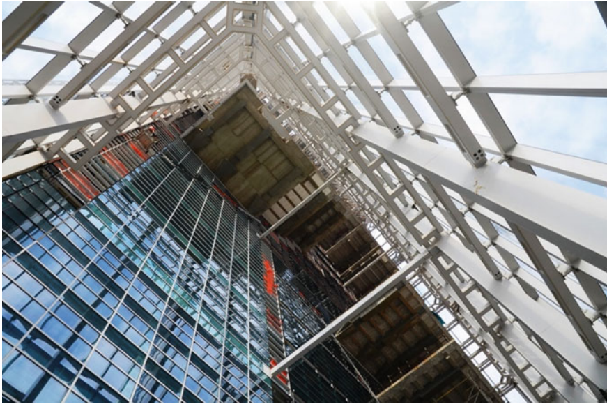
Fig. 1.7 Massimiliano and Doriana Fuksas, Regione Piemonte headquarters, Turin. Interfaces between the elevation framework, vertical and horizontal, and the frame profiles connecting to the perimeter enclosures, according to connections directed to accentuate the exposure of the supporting elements towards the outside. © Courtesy of Schüco
