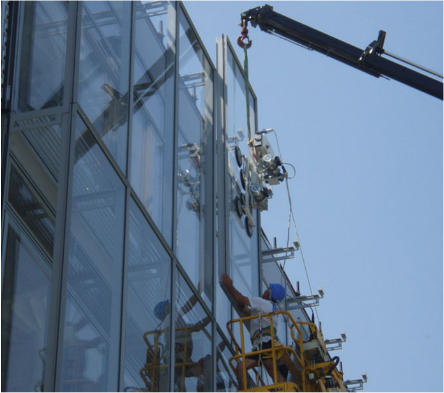
Fig. 4.22 Maurizio Varratta, iGuzzini Lab , Recanati. Application of the external skin to the main curtain wall, reducing wind pressure and allowing the opening of windows relative to the internal section (even at high levels of the building). © Courtesy of Pichler Projects
