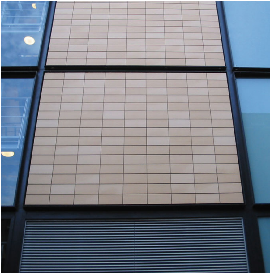
Fig. 1.15 Nicholas Grimshaw and Partners, University College London's New Engineering Building , London. Archetypal suggestions of traditional materials in the façade: perimeter texture in aluminium profiles supporting brick and double-glazed modules and bands. © by the Authors
