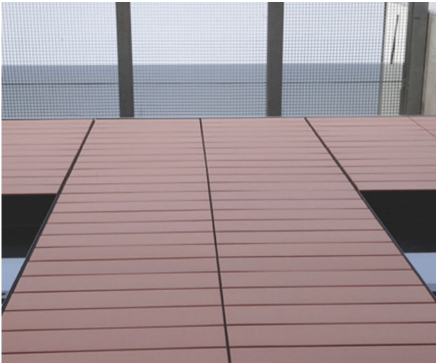
Fig. 1.16 Integration between the envelopment in terracotta elements, the transparent surfaces and the “ephemeral” projection of the upper grid of the Piterak system: expressive consolidation of morphological and material connections in the systemic articulation between structures of different tectonic invoice. © Courtesy of Terreal
