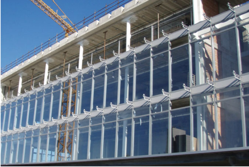
Fig. 4.21 Maurizio Varratta, iGuzzini Lab , Recanati. Building of the internal curtain wall system, consisting of double-glazed sheets, in order to avoid the phenomena of both surface condensation of water vapour and overheating. © Courtesy of Pichler Projects
